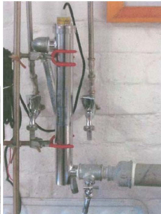
Figure 3: UV disinfection device with discharge pipe
